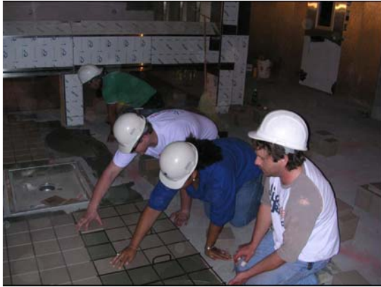
Patrick Beckham and Casera Sparks volunteer to lay tiles in the kitchen floor of West Cobb High School.
