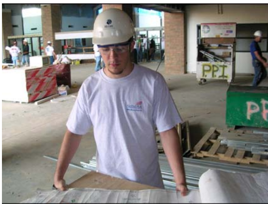
Dakota Burgener looks over the drawings for the details going into the upper floor atrium.
